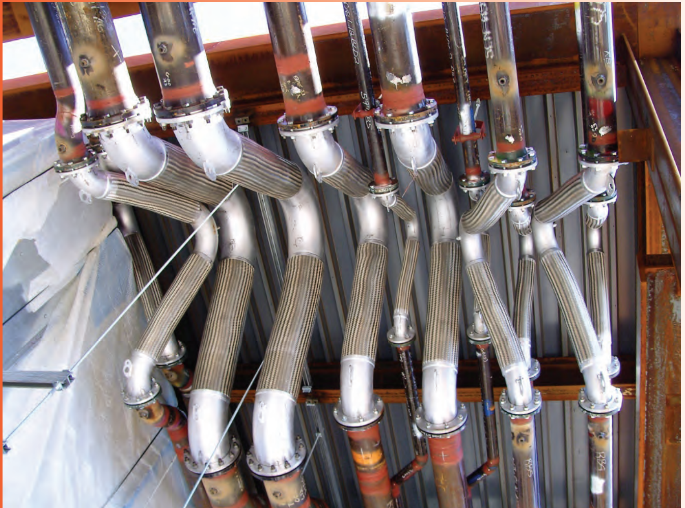
VERTICAL VFL INSTALLATION (Apex Near Ceiling)
